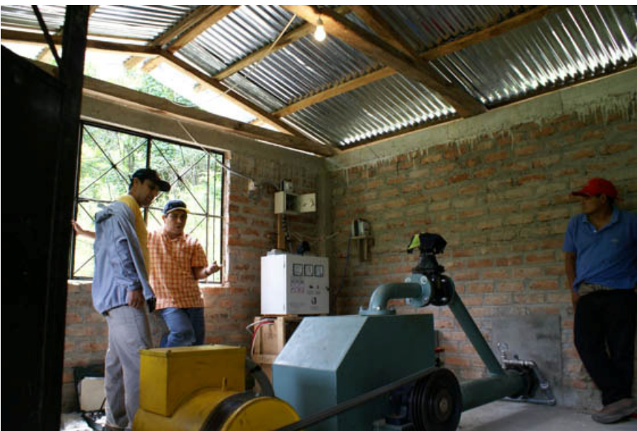
The interior of the generator house with Pelton wheel, generator and control equipment
